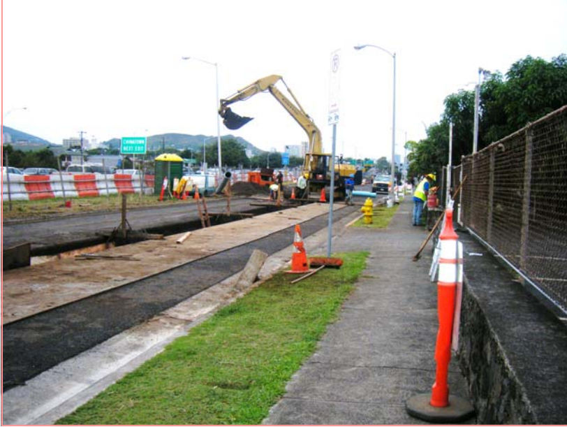
Ideal Construction crew working on the area in front of the shrine
